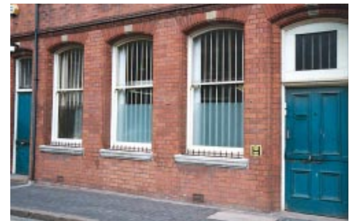
Internal security grilles
