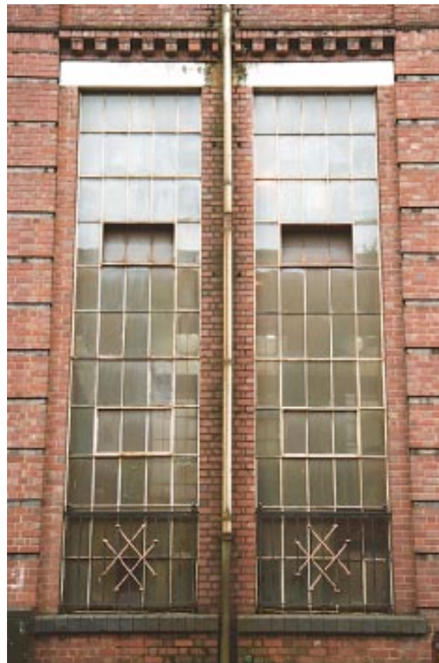
External demountable security grilles
