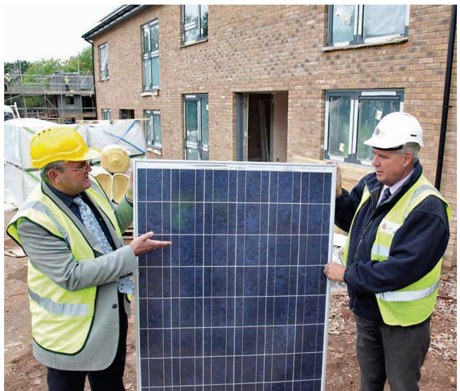
New housing with solar panels
