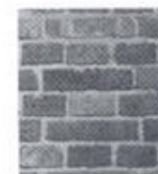
Beautifully crafted brickwork in English bond - alternate rows of 'headers' and 'stretchers'.
